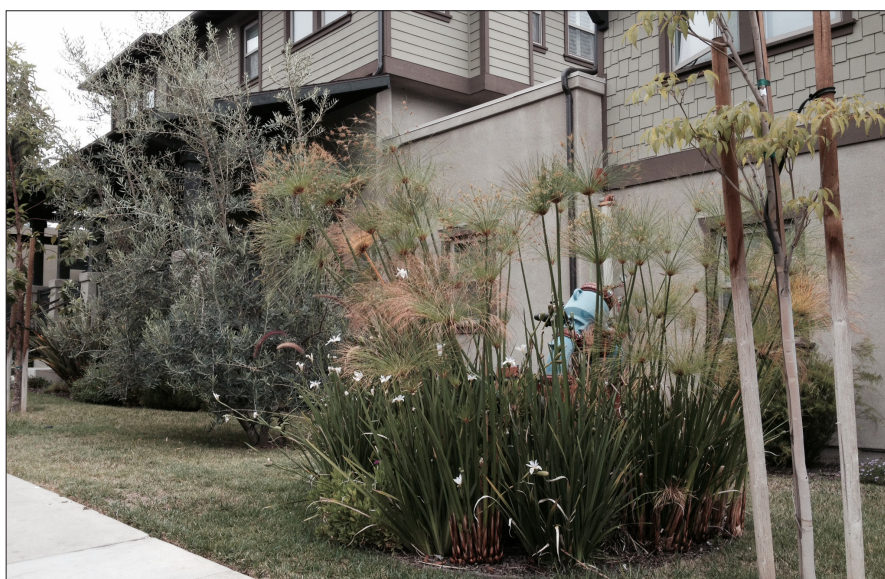
A back flow preventer that is located immediately adjacent to the building and is screened from the view of the sidewalk and street by shrubs.
