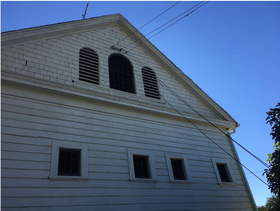
Photograph 8: Northwest elevation of the carriage house with wooden siding and windows visible, flaking white paint, camera facing south, January 9, 2009.
