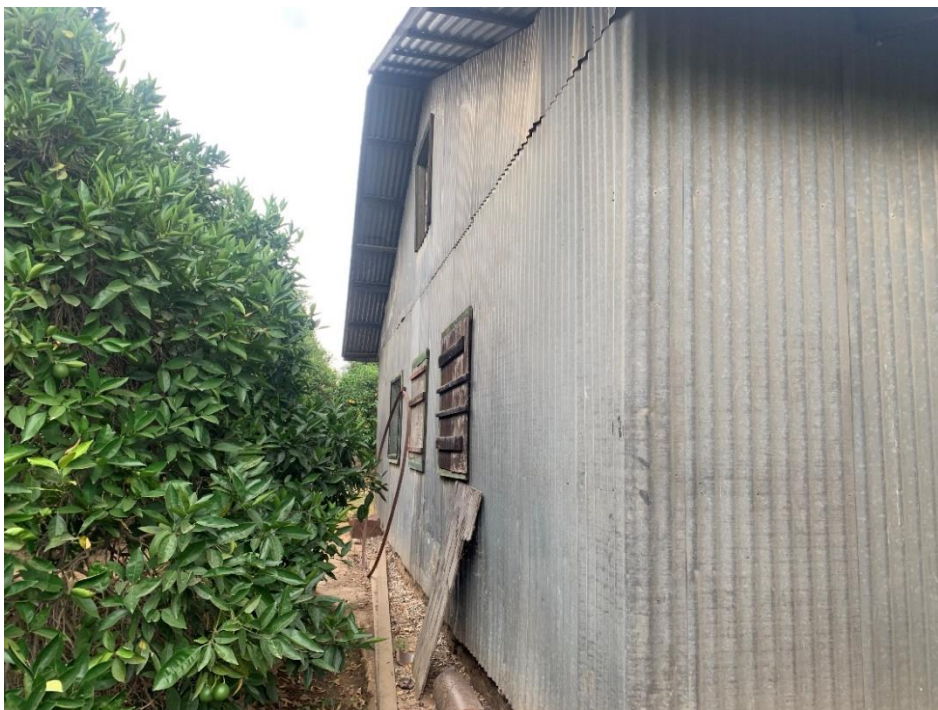
Photograph 3: View of rear northeast elevation of the garage, rear windows covered by wooden boards, camera facing southeast, July 25, 2019.
