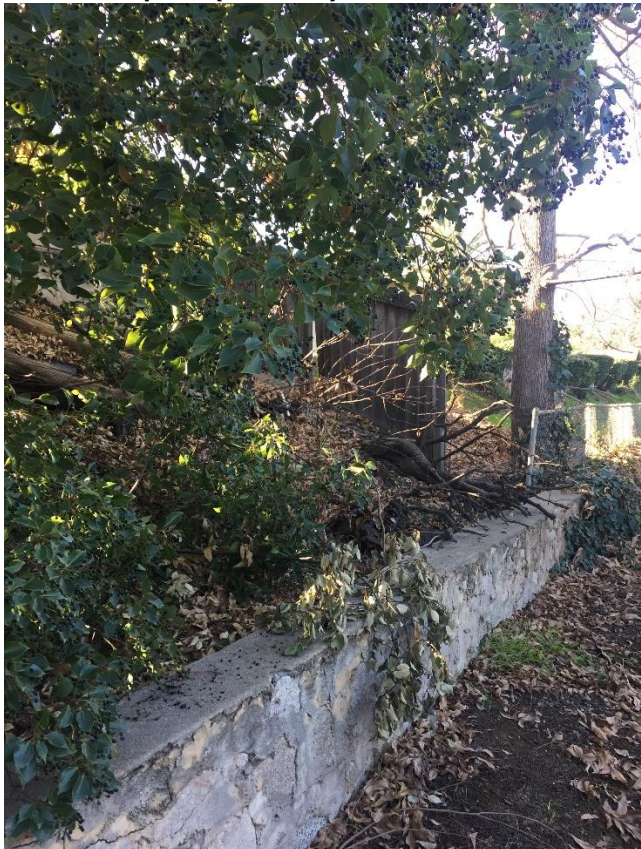
Photograph 2: Detailed view of the concrete masonry footing along the southeast boundary, January 28, 2020.
