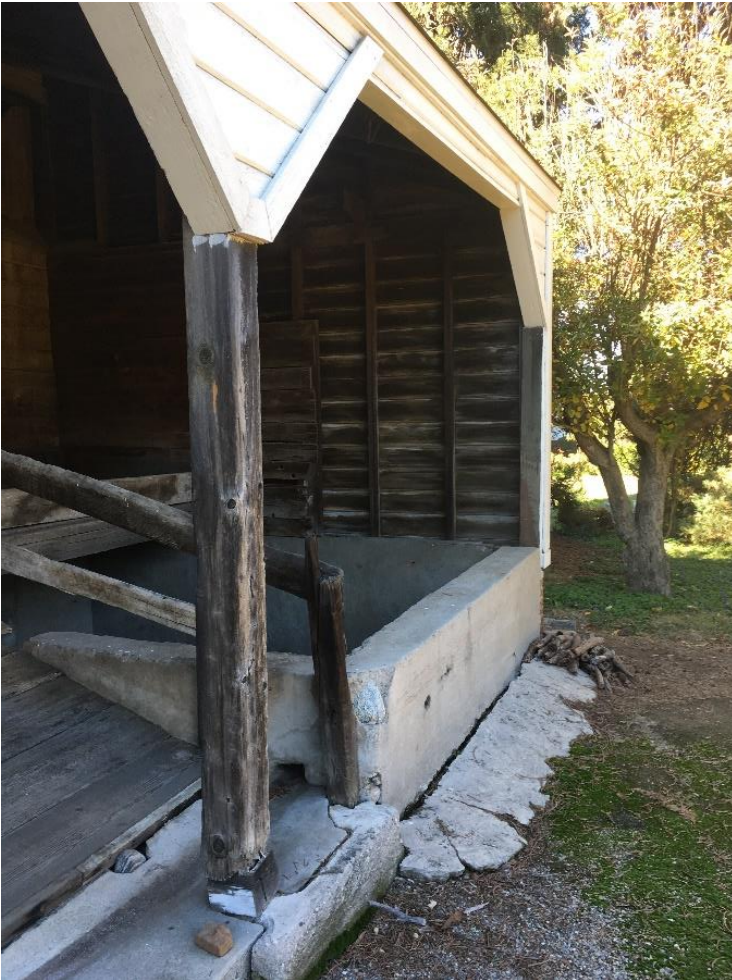
Photograph 6: Cement basin adjacent to wooden entryway in northernmost corner of the carriage house, January 9, 2019.
