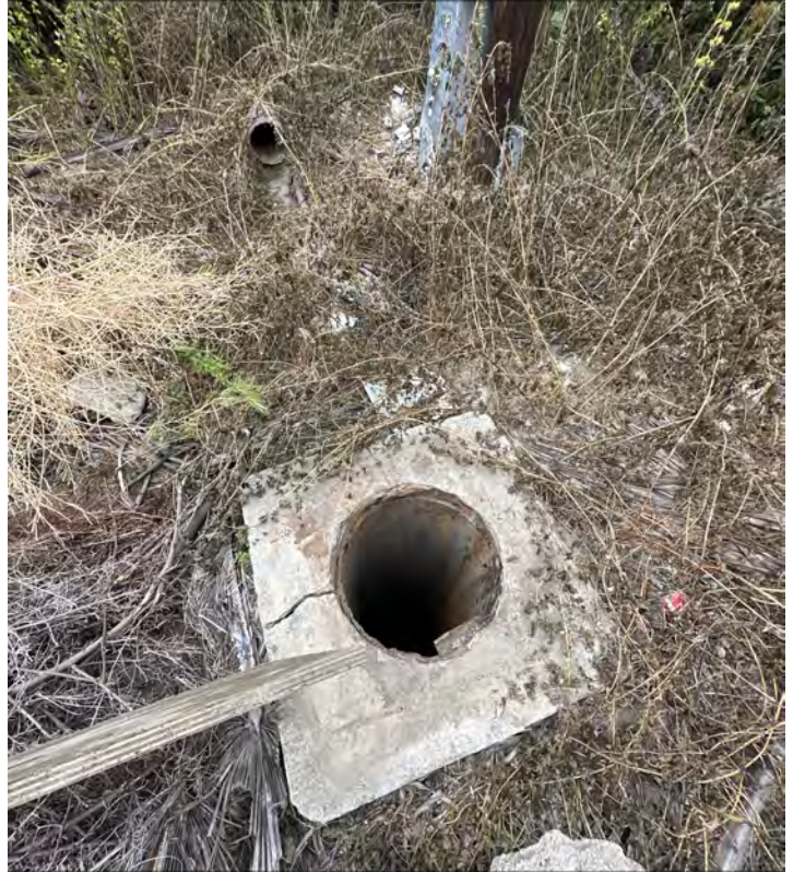
Well in NE Corner
