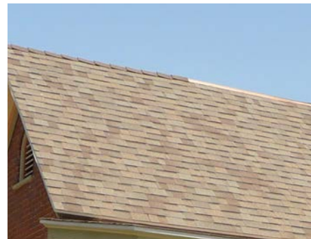
Reattach or replace loose or missing shingles.
