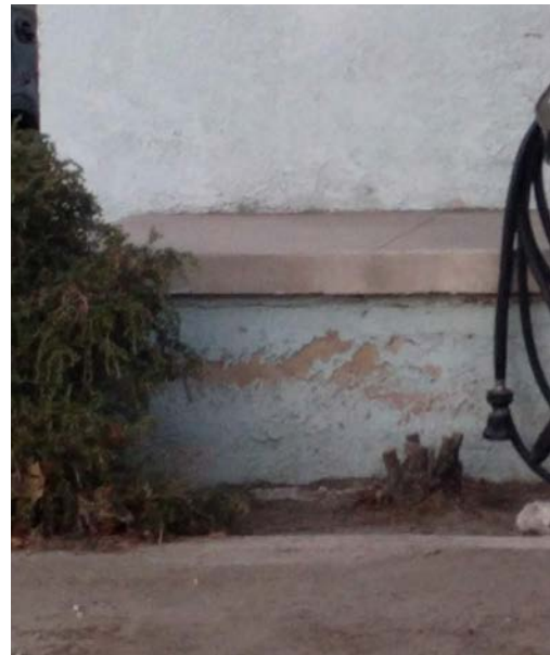
Weathered stucco at a porch.
