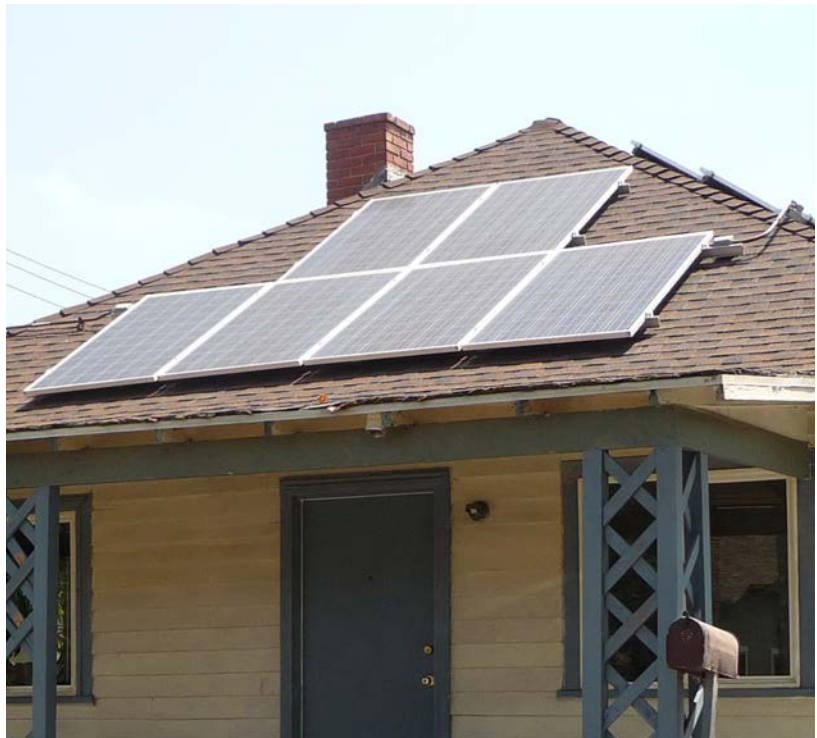
Solar panels on a composition shingle roof.
