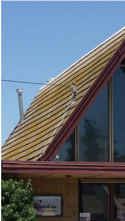
Biological growth on a wood shake roof.
