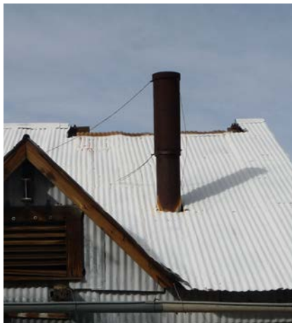
Corrugated metal roof with open hole.
