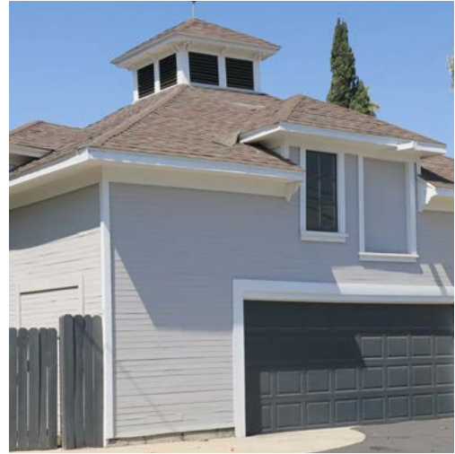
Restore a historic ancillary structure's missing components, such as historic garage doors or infilled openings.
