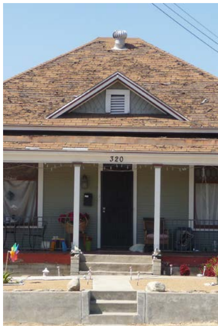
Deteriorated asphalt shingle roofing on the former Harbert Residence (1907).
