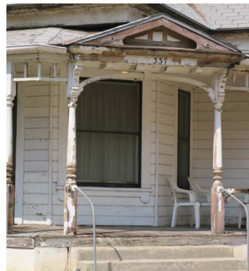
Deteriorated woodwork at a porch.
