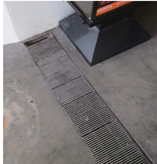
Drain with uneven grate panels.
