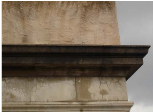
Repair and maintain historic architectural features, such as this cornice, to prolong its life.
