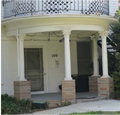
Restore non-historic porch components, such as these piers supporting original porch columns, to their original condition.
