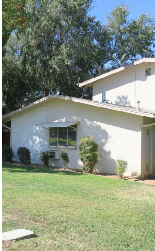
An example of aluminum slider windows, typical of Redlands' postwar multi-family development.
