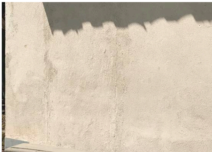
Incompatible stucco at an infilled door.
