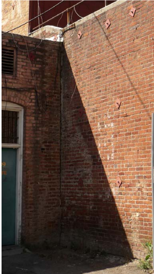
Efflorescence on a historic brick wall.
