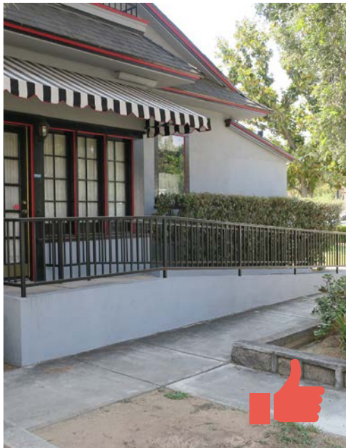
The accessibility ramp at the side of this building is painted and retains a simple design that is compatible with the historic building.
