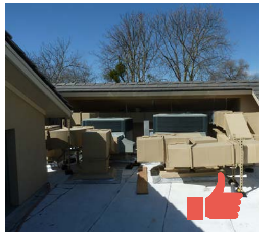
This mechanical equipment is located below the parapet of the building so that it is not visible from the public right-of-way.
