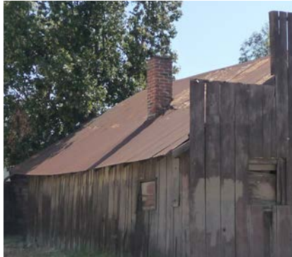
Corroded and warped corrugated metal roof.
