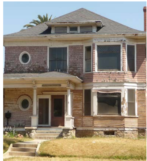
Weathered paint on exterior woodwork.
