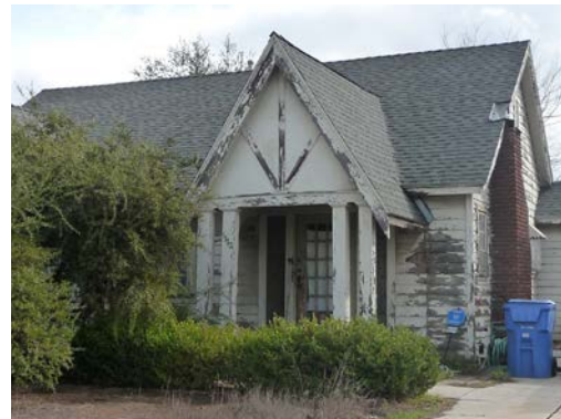
Poorly maintained wood cladding and trim.
