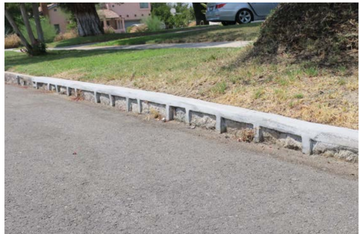
Inappropriate concrete repairs to cut stone curbing.
