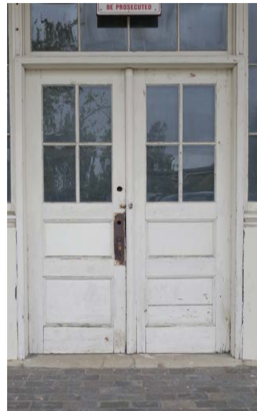
Weathered doors with corroded and missing hardware.
