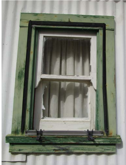
Weathered and racked window needing repair.
