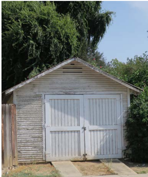
Routine maintenance, such as painting, is important to the preservation of a historic ancillary structure.
