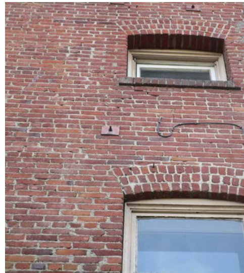
An example of seismic anchor plates that blend in with the surrounding brick.
