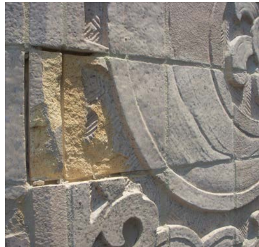
Damaged terra cotta detail.
