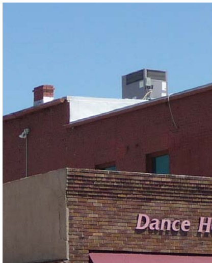
HVAC equipment atop a commercial building.
